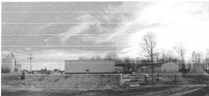
Progress on the Fleet Maintenance Building Expansion. The concrete floors have been poured and the block wall has been completed.
