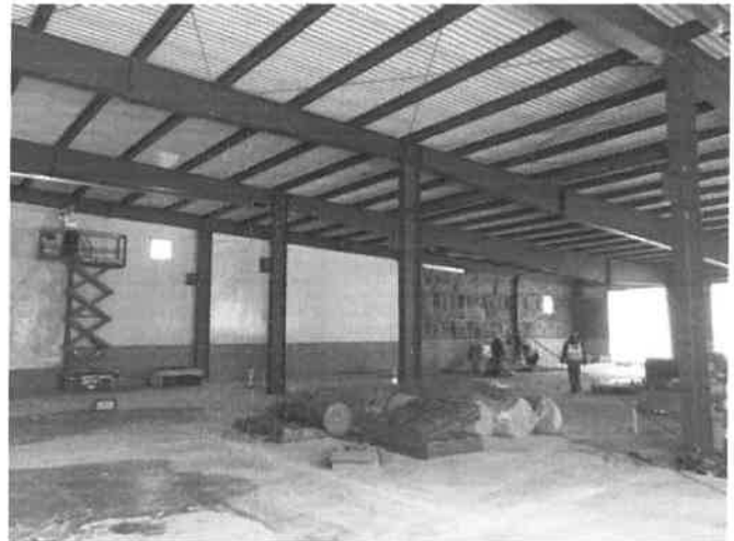
The 9" layer of brown insulation has an R-factor of 30. It's placed against the outside steel wall, followed by a vapor barrier, followed by white metal siding. When all is finished, we'll have a well insulated building.
