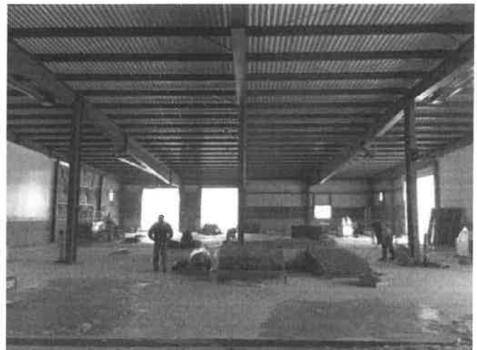
Dave Bonthuis, Wastewater Maintenance Supervisor, views with pleasure the progress on the new building.
