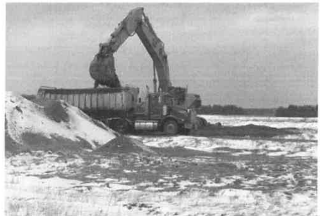
This month Yellow Rose Trucking began hauling sludge from the sludge drying beds to the landfill after the Board of Public works awarded them the sludge hauling bid at the February Board meeting. The Wastewater’s heavy equipment operator, Chris VanderLaan, is doing the loading. The sludge drying beds are converted RI beds. They are not concerned in our current RI renovation, as they are no longer used to treat water.
