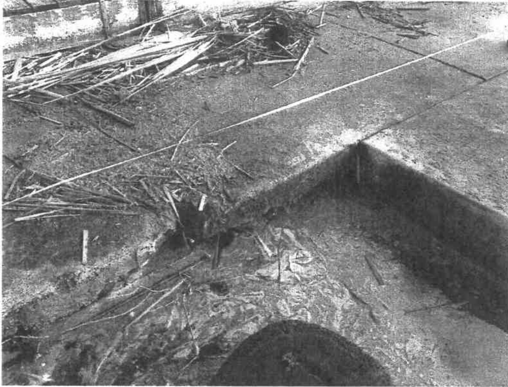
Main Pier— Concrete damage at stairs (12/2020)
