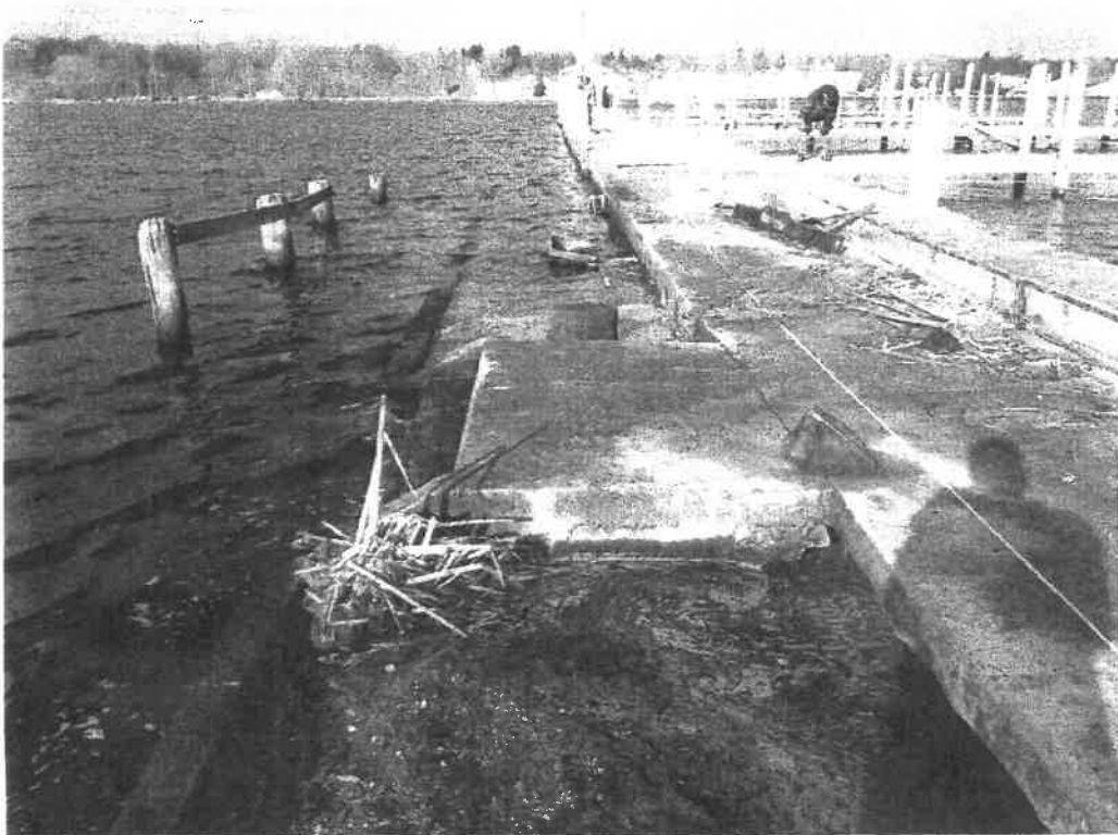
Main Pier—Most extreme settling north side of stairs (12/2020)
