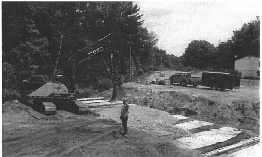
Construction activities at Sweeter Road and Little Cedar Creek crossing on June 6, 2023.
