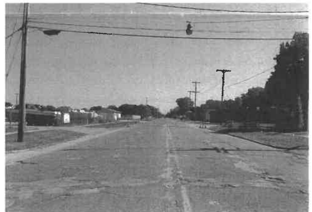
Work began this summer on this stretch of Broadway Avenue in the City of Muskegon Heights.
