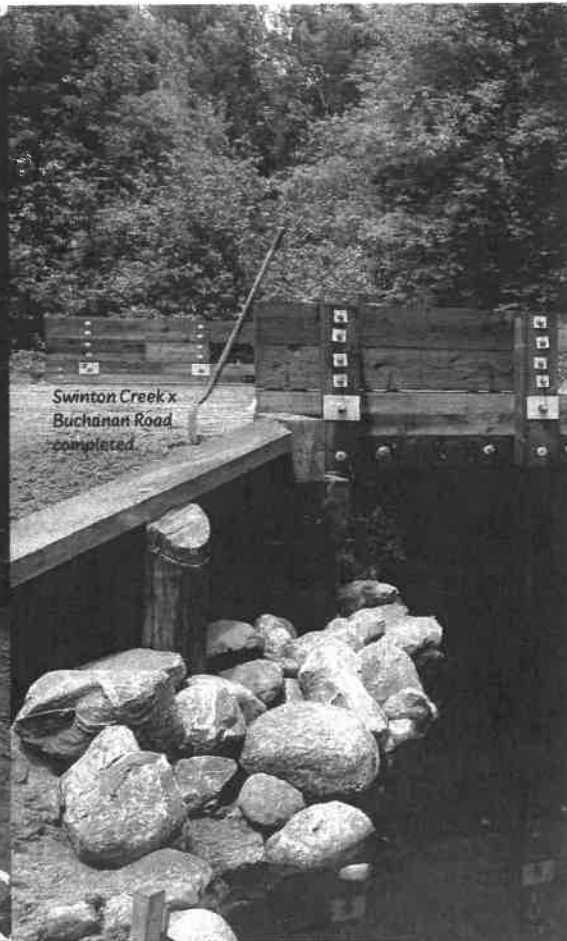
Viewpoint of the Stony Creek habitat restoration from the new timber bridge. The open area past the rock will be the location of the access pier.
